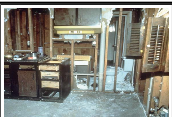
Structural flood damage includes broken walls and damage to insulation and wallboard
